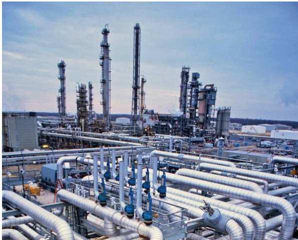
Industrial Utilities & Processing Plants
